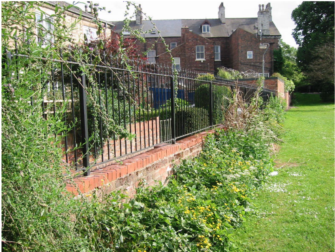
c) Boundary wall and railings – looking in a southwesterly direction towards the back of properties on Scarcroft Road.
